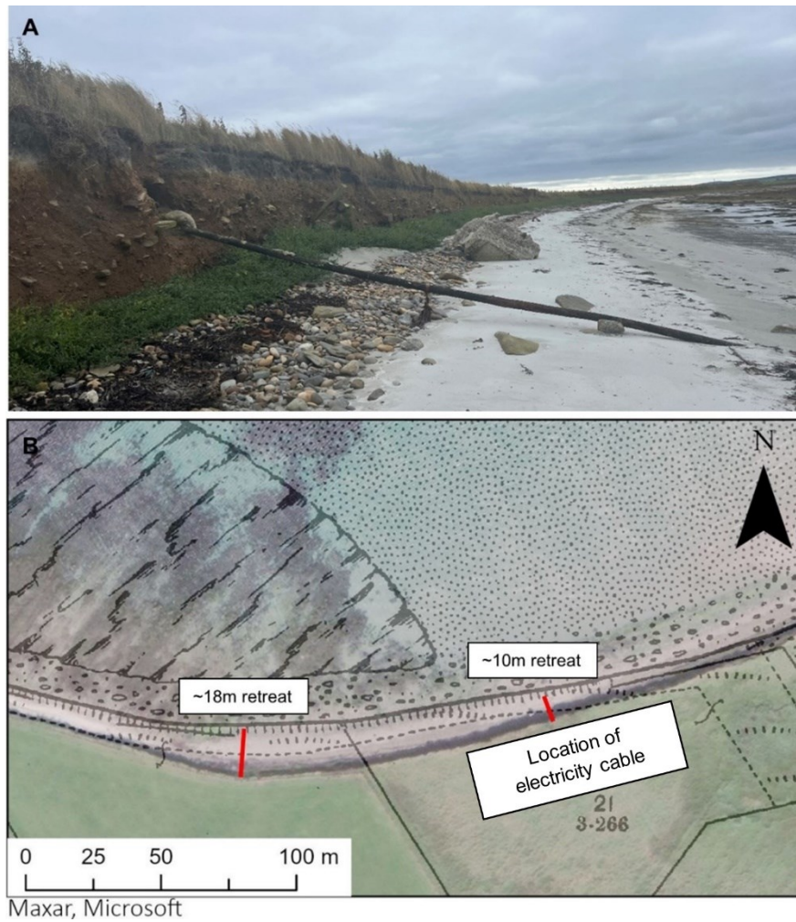
Figure 6A. Submarine mains electricity cable exposed from eroding coast edge, Sands of Odie. Figure 6B. Comparison of coast edge using modern satellite imagery and 1900 historic mapping (1:2500 County Series 1 st Revision [TIFF geospatial data], Scale 1:2500. Tiles: orkn-hy6229-2.tif, Updated: 30 November 2010, Historic, Using: EDINA Historic Digimap Service, https://digimap.edina.ac.uk , Downloaded 2023-10-09).
